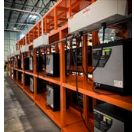
Battery Chargers & PDP Panels
