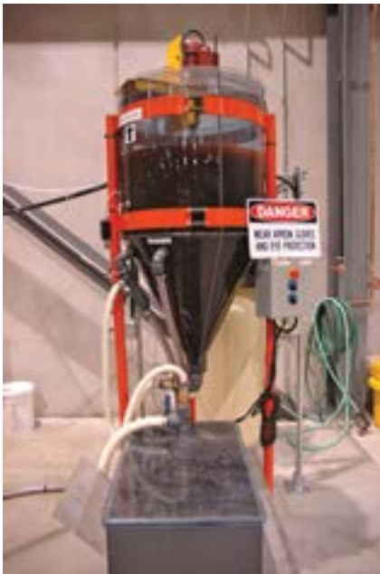
WWTS - filled with waste water and in operation
