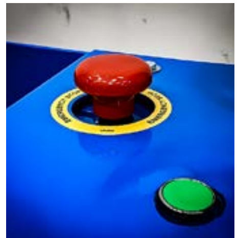
Emergency stop controls
