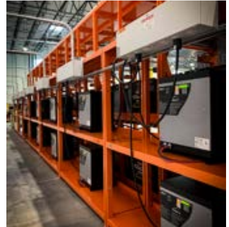
Battery Chargers & PDP Panels
